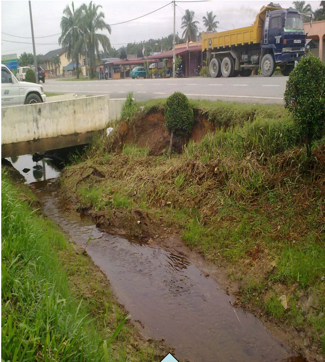
Tebing mudah runtuh
